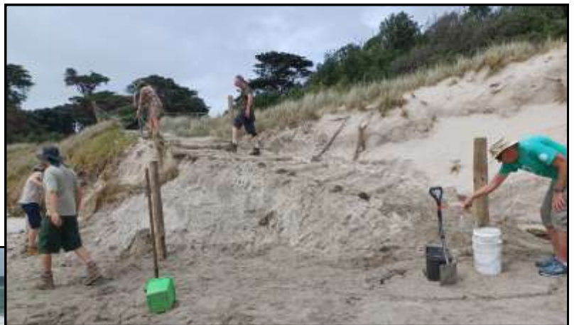
The final filling still had to be done by hand, with buckets and shovels.
