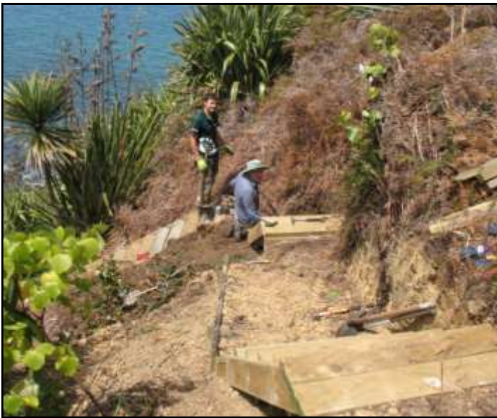
Thursdays volunteers repair their recently built Maori Bay Track by installing steps across a recent slip area.
