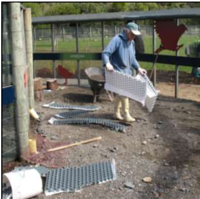
Volunteer Ron Dyer installs the foundation flooring for the koru planting and interpretation display as this project nears completion.
