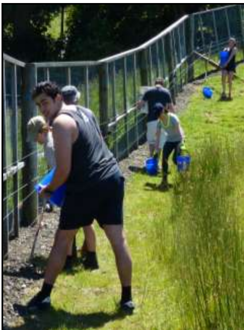
Volunteers from Pricewaterhouse Cooper strengthen the base of the Pest Proof fence with metal.
