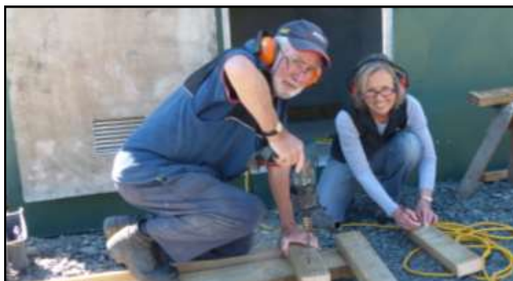
Volunteers Roger Williams and Karen Hoksbergen build shelves for the new chemical shed.
