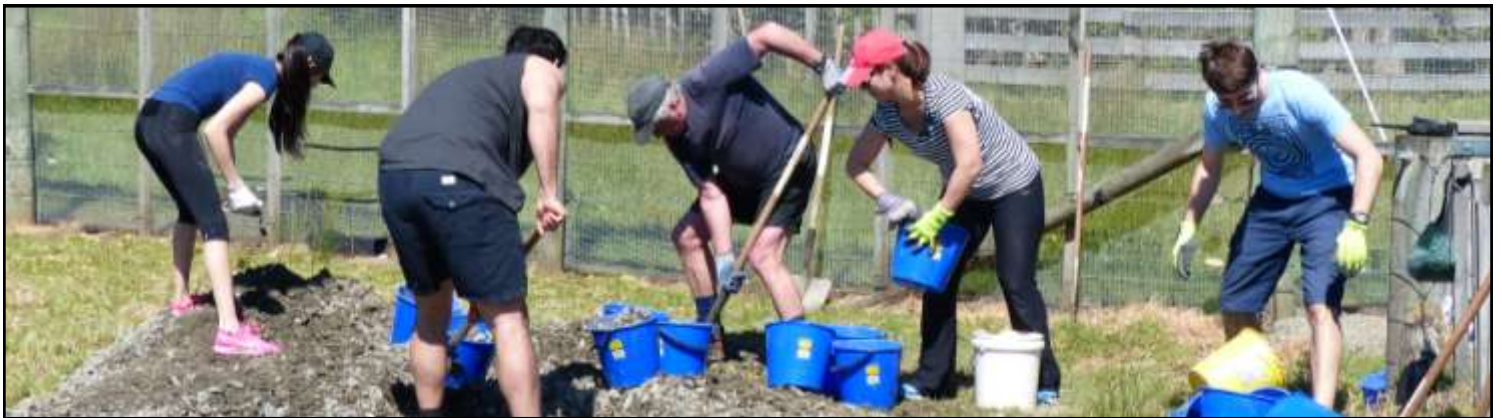
Mark Paterson helps volunteers from Pricewaterhouse Cooper load buckets of metal for dispersal along the PP Fence.
