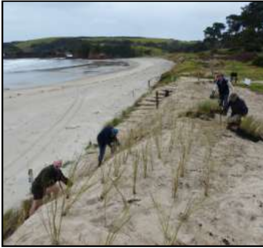
A clay cap is to be progressively removed from the dunes at Anchor Bay as it enables the sea to erode beneath it. Volunteers plant the first section with spinifex to prevent erosion.
