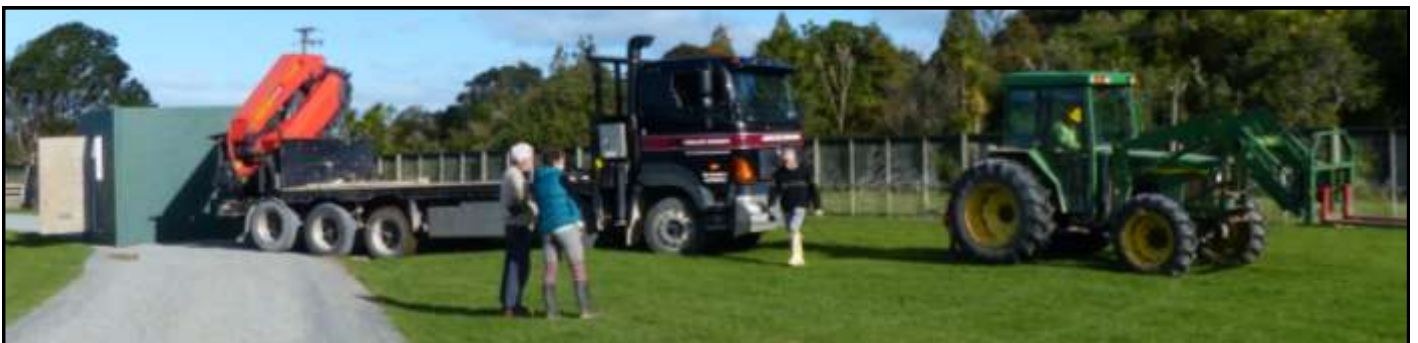
A new chemical shed arrived to go in the workshop yard. Roger Williams and Sharon Kast assess the situation as the truck gets stuck, the chemical shed is placed on the access road and the farm tractor is employed to get the truck moving again.
