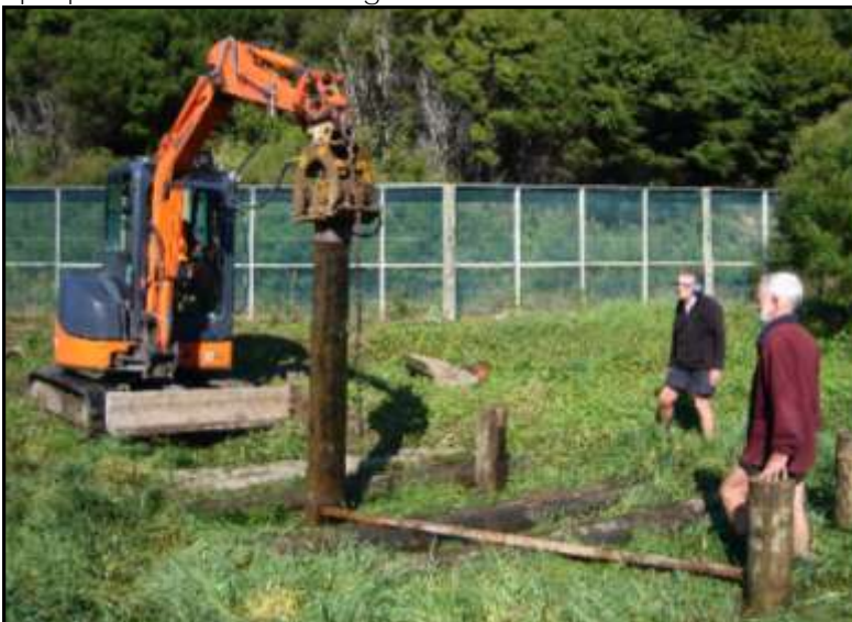
Mangatawhiri boardwalk will complete the Mangatawhiri loop Trail. Poles are sunk for construction.
