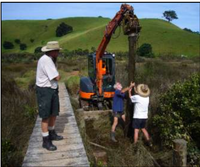
The lagoon boardwalk will become part of the new Heritage Trail. Foundation posts are lowered into position alongside the old bridge which will later be demolished. Photo. Right. Poles are cut in preparation for attaching bearers.
