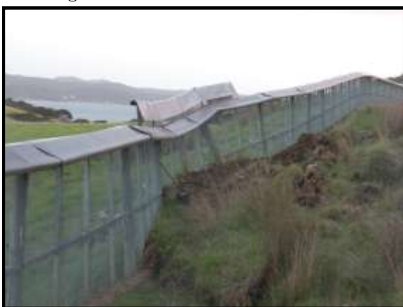
Above. For nearly a week the impressive temporary repair protects the sanctuary from predator incursions.
