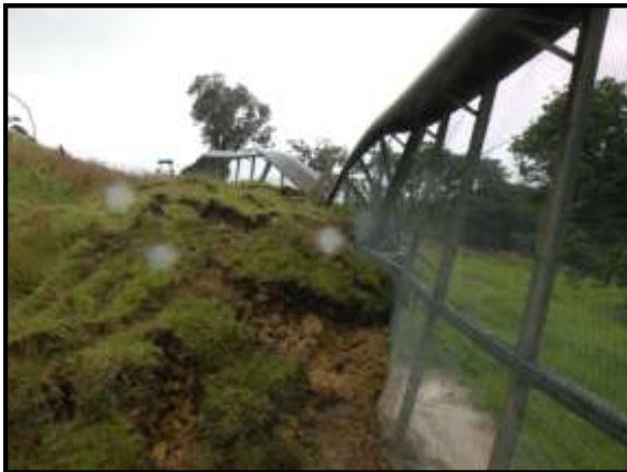
Cyclone Wilma slams the Warkworth area and sends a slip on to the pest proof fence causing a serious breach.
