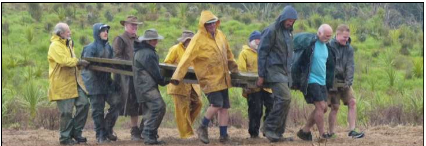
If the bridge needs shifting and there is no tractor and front end loader available just pick it up and shift it!
